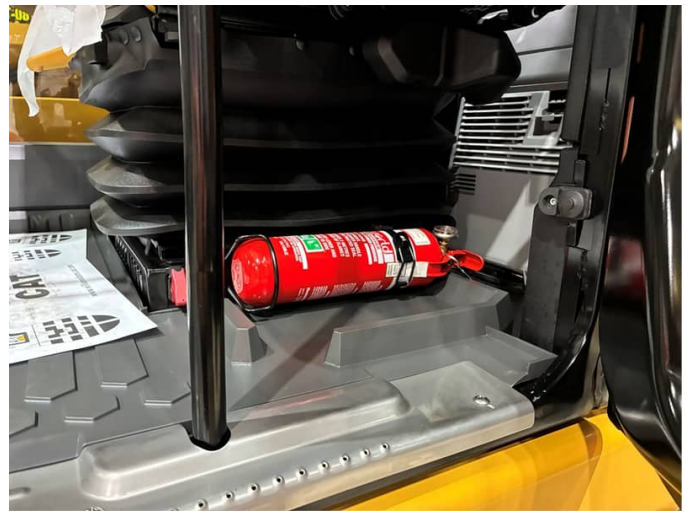
1kg extinguisher in operator compartment.
