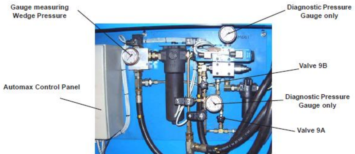
Figure 9g Dumpy Jack Circuit Shut Off Valves
